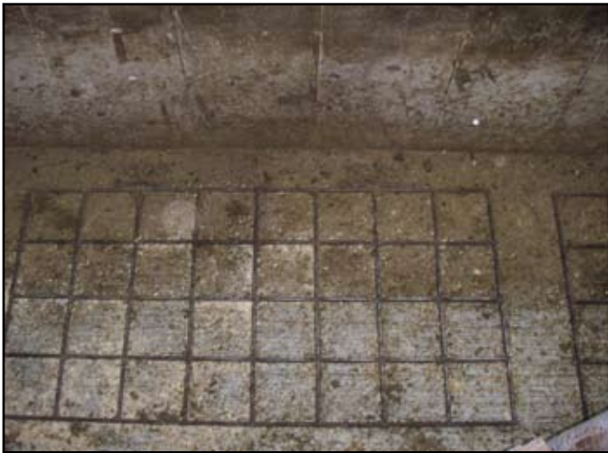
Photo 13. Hinged floor grating lifts for cleaning.
